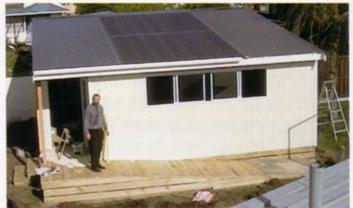
■ Roof-integrated photovoltaic modules on the Vardon School in Hamilton.
