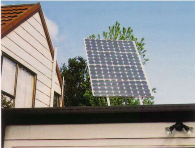
■ An array of four 75W monocrystalline modules mounted on a roof top.
